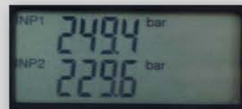
Screen shot showing two inputs. Pressure 1 and 2.
